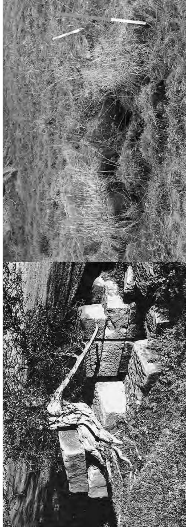
Plate 5 Destruction of a formerly well-preserved sandstone sluice housing at Willows Farm, due to encroachment of tree roots (image on left dates from 1991; courtesy of Mr Andrew Allen; image on right dates from 2008, during field survey)
